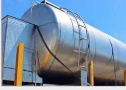
16 DEPOLAMA TANKLARI STORAGE TANKS
